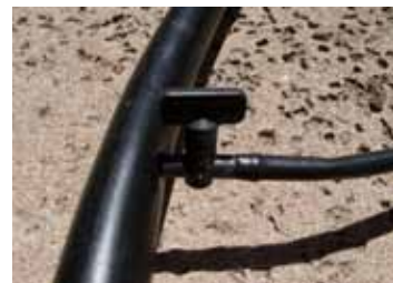
Valve inserted in 1/2-inch tubing
